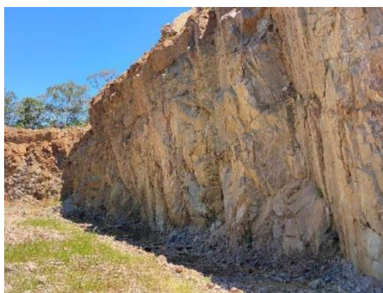
Photograph: 13 – existing quarried face viewed south-west showing over-hang due to defect orientation.
